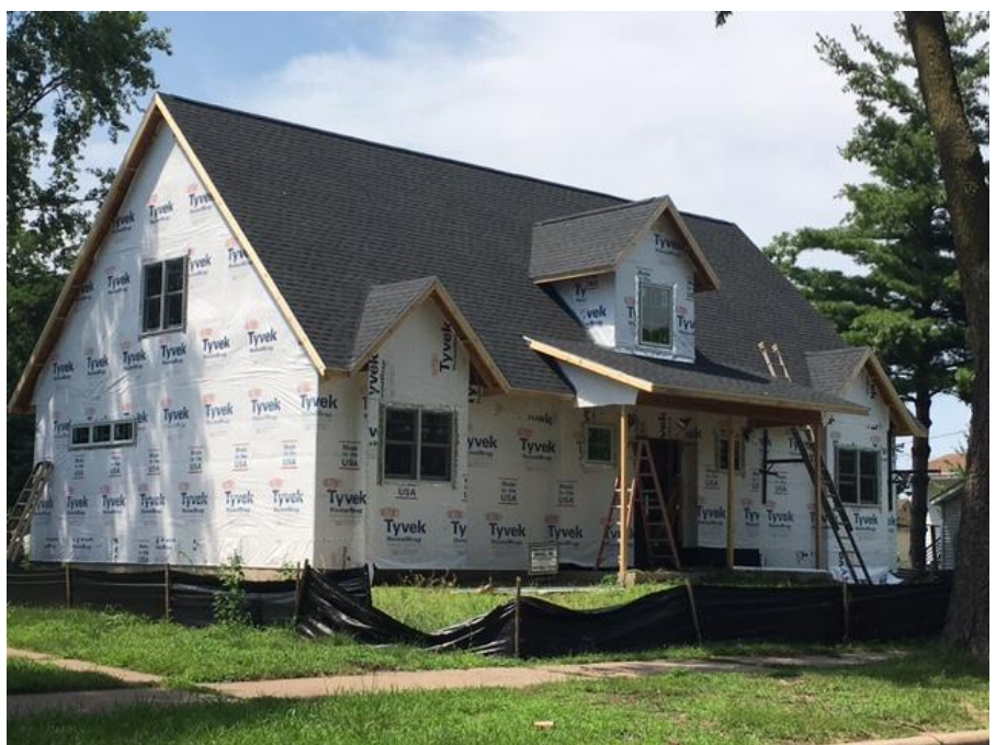
Above is a Promise home on 5th Avenue (above), which is coming along nicely and will be complete soon for a private homeowner.
